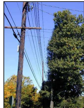
Best compromise possible? Good utility pruning for the wrong tree in the wrong place.
